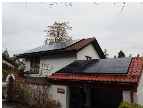
Rooftop PV system 9,81 kWp with smart PV inverter equipped with autonomous Volt/VAr and Volt/Watt control functions
