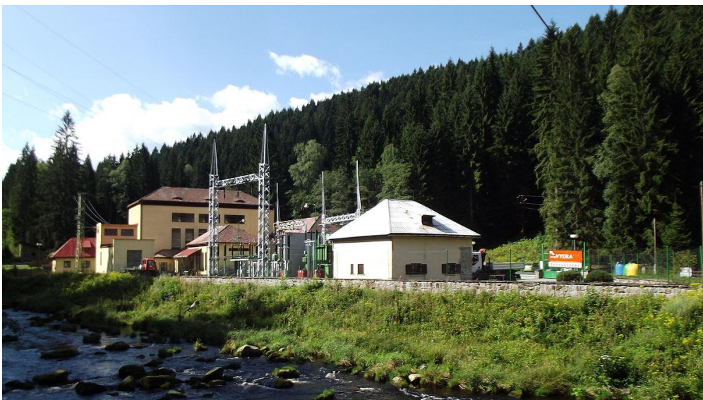
Small hydro Vydra with 6,4MW of installed capacity
