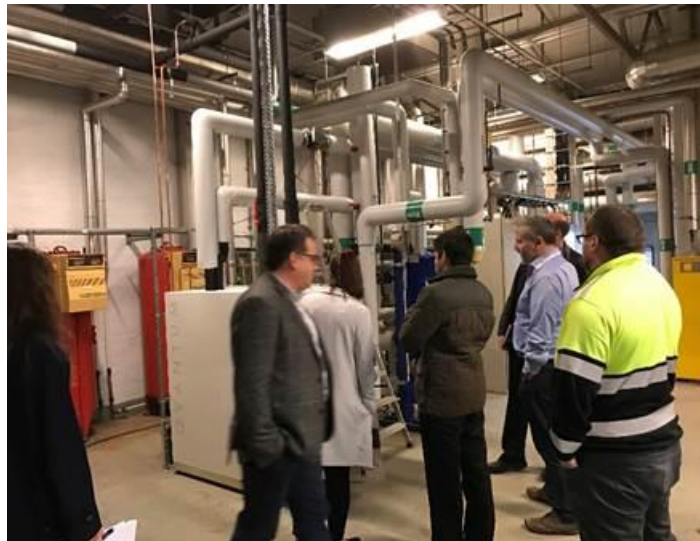
Heat pump at demo site in Malmö
