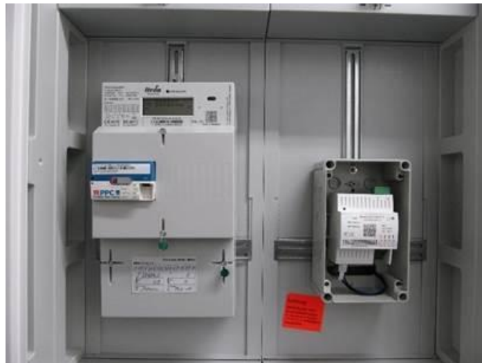
Smart meter with smart meter gateway and the control box to be tested in InterFlex
